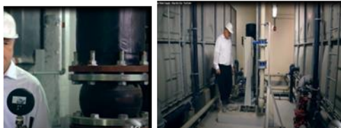
Fig 37: Water flow from the main pump to the last reservoir
